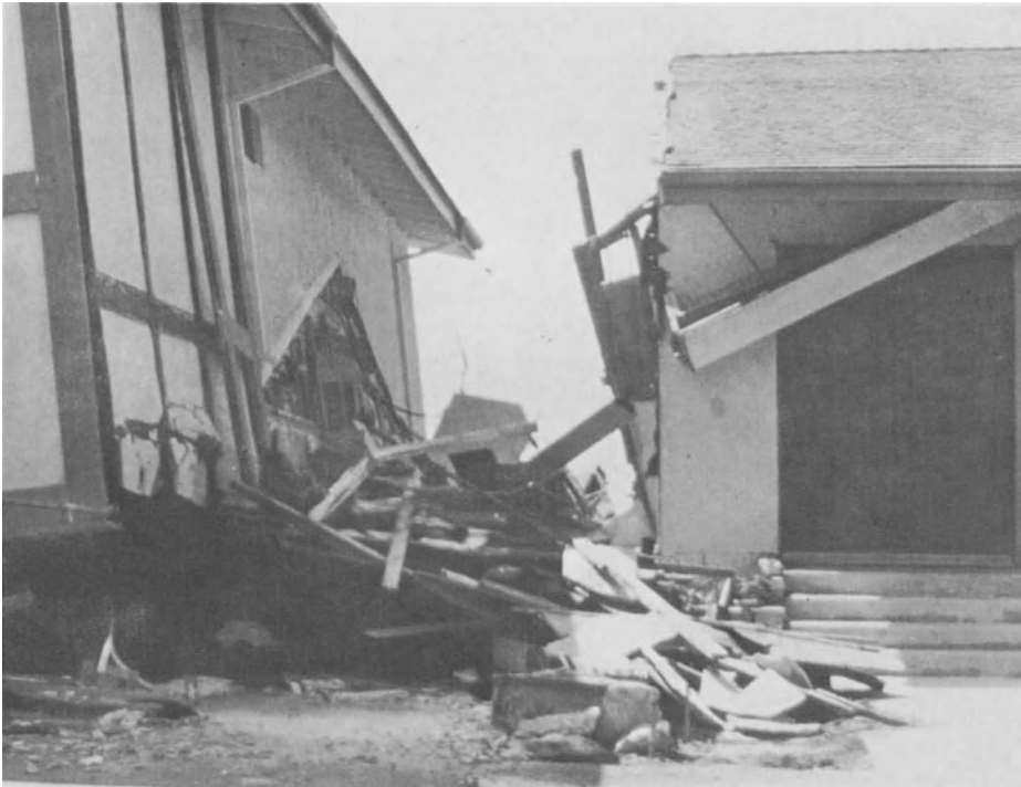
Plate 1.7. Two-story wing of a new split-level house collapsed in the 1971 San Fernando earthquake crushing the automobile parked in the ground-level garage. The garage construction used reduces the lateral bracing. (Photo by B.A. Bolt)
