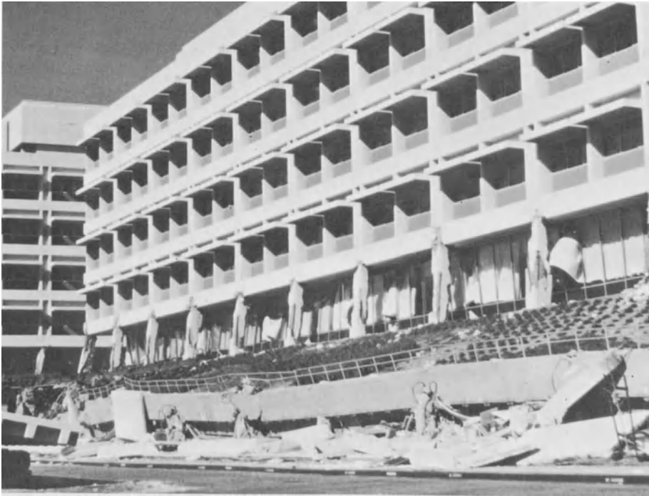
Plate 1.6. Damage to reinforced concrete columns at the new Olive View hospital in the 9 February 1971 California earthquake. (Photo by B.A. Bolt)
