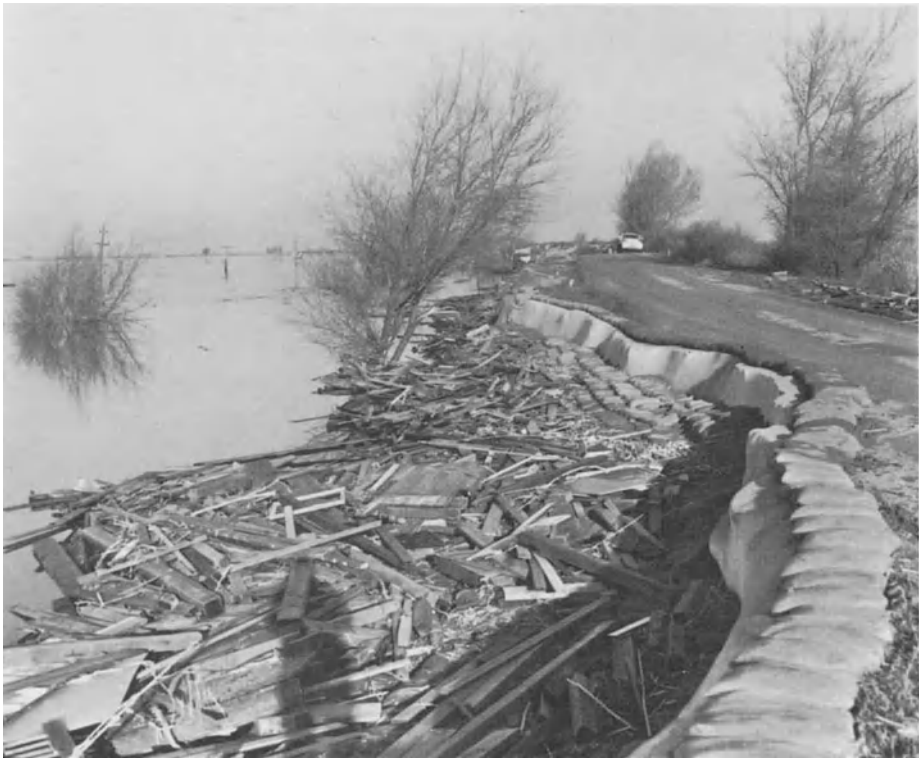
Plate 7.9. Repair work to levee along Sherman Island, California. (Courtesy of California Department of Water Resources)
